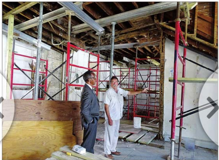
INSPECTION — Mark Shuttleworth, right, and Vernon Burton, vice mayor of Lake Helen and a member of Greater Union First Baptist Church, examine the original wooden beams that hold up the roof of the J.W. Wright Building, surrounded by bolsters that hold up the ceilings. One such original wooden beam, on the west side of the building, is a whopping 35 feet long. Restorers were surprised to find the 6-inch-by-11-inch heart-pine beam was in excellent shape.
